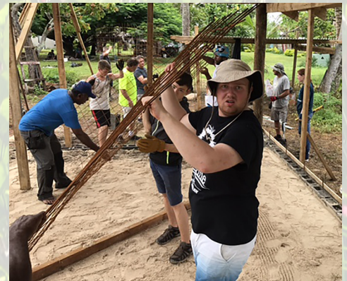
Ian Griffith, a GSAA alumnus, helps lay the iron bar for the church floor.
